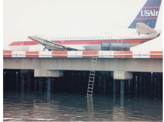
LaGuardia Airport used the SeaShield Series 100 System to provide corrosion protection for over 2,000 steel piles.
