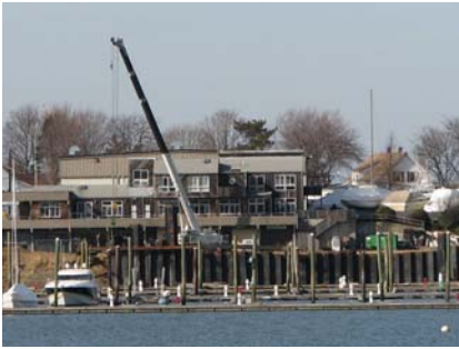
Tern Harbor Marina in Weymouth, MA where the old corroded timber was replaced with new Rigspray coated steel sheet piles.
